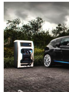
Rapid 50kW charger
