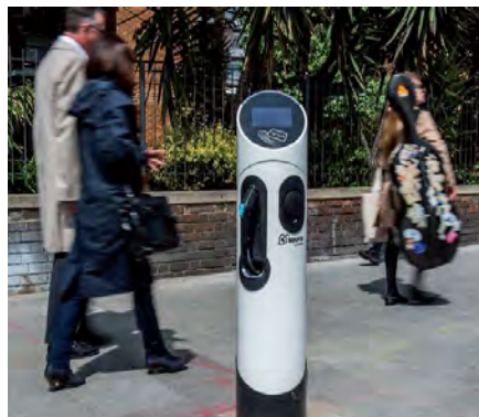
7kW charging point post
