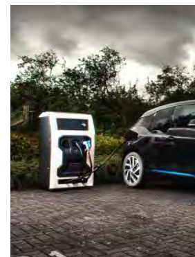
Rapid 50kW charger
